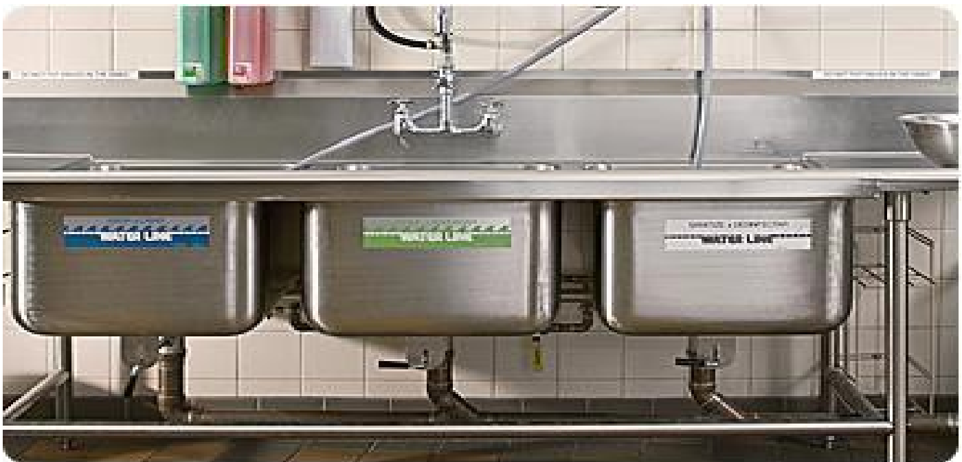
Figure 7: Three compartment sink
