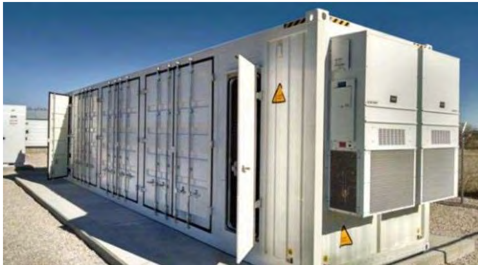
Figure 5-10 Representative Battery Storage System Enclosure (Exterior View)
