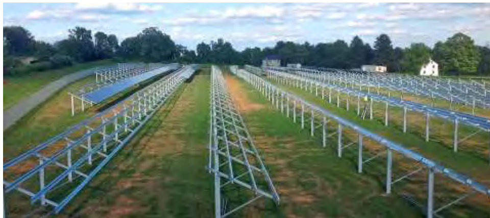
Figure 5-5 Representative Fixed Tilt Installation (Side View of Racking and Modules)
