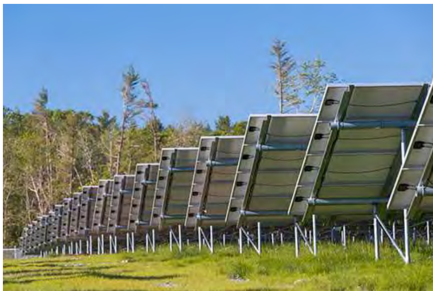
Figure 5-6 Representative Fixed Tilt Installation (Back View of Modules)
