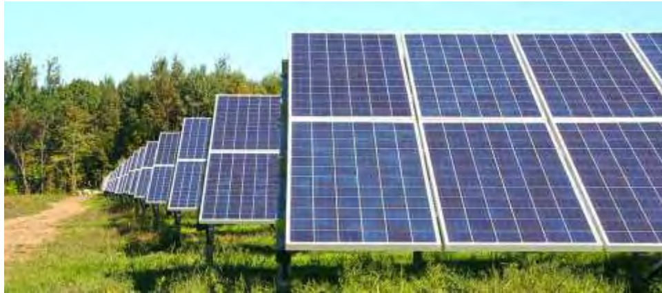
Figure 5-4 Representative Fixed Tilt Installation (Front View of Modules)
