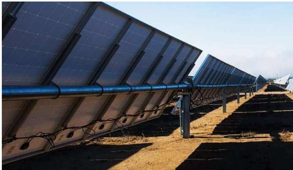
Figure 5-8 Representative Single Axis Tracker Installation (Back and Side View of Racking and Modules)
