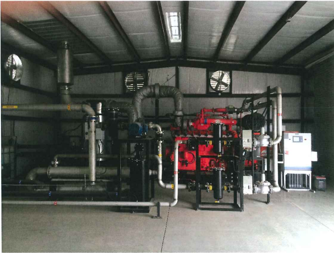
Figure 2: Inside Metal Building, looking at engine and genset
