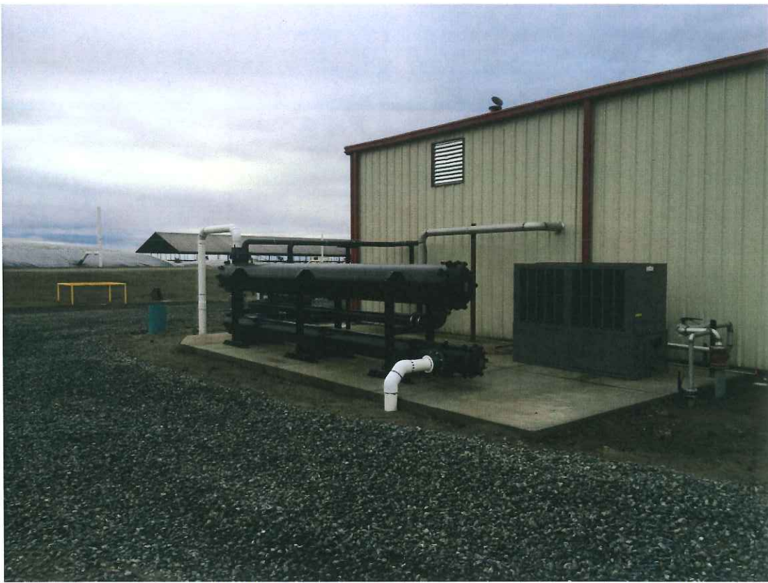
Figure 1: Metal Mechanical Building with gas conditioning equipment slab
