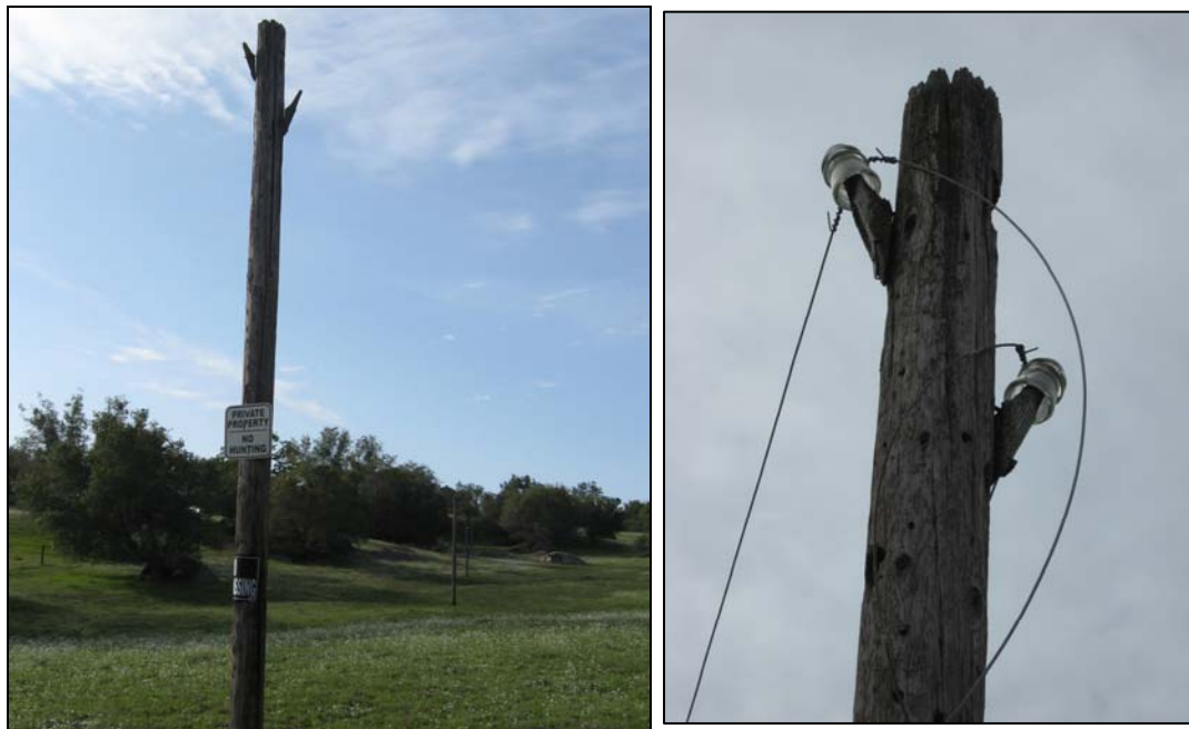
Figure 3.8. Overview (left) and close-up of glass insulators at PL-Mad-003.
