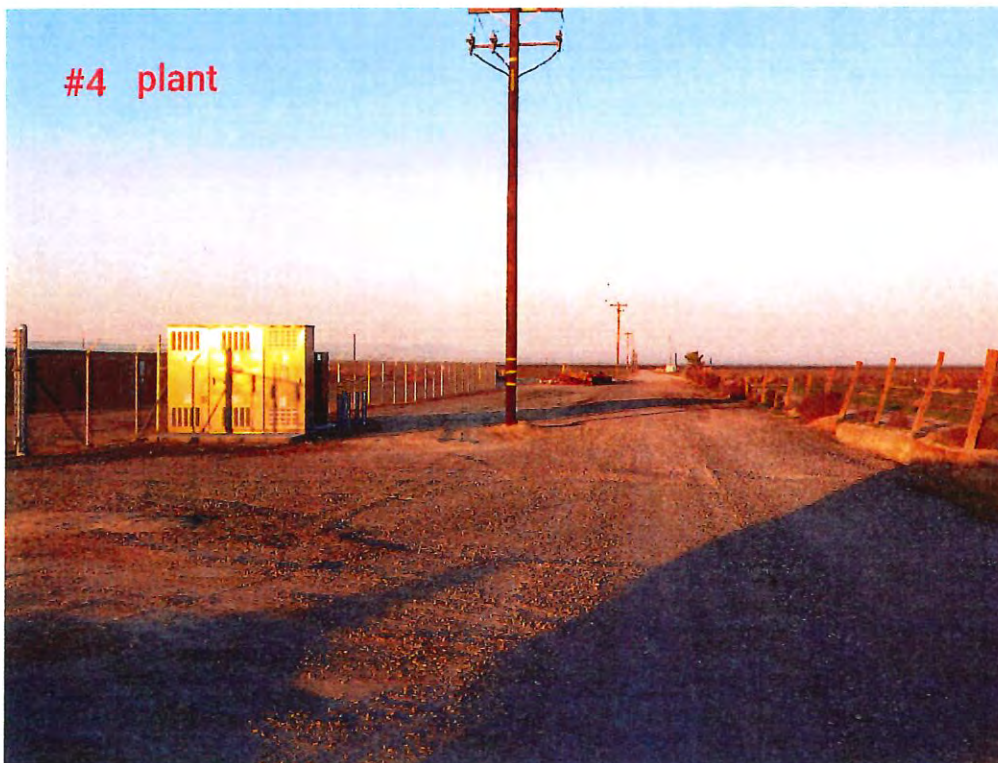
Photograph 4: Looking west along northern property from the northeast corner of the solar array in APN 41-172-04.
