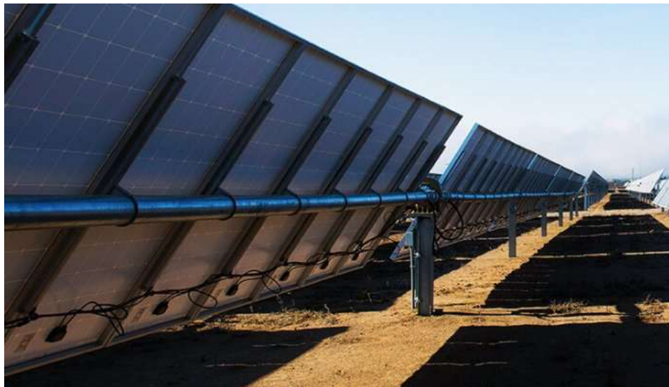
Figure 5-8 Representative Single Axis Tracker Installation (Back and Side View of Racking and Modules)
