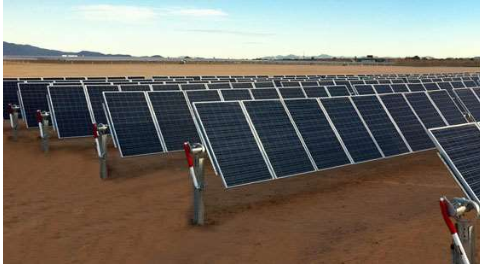
Figure 5-7 Representative Single Axis Tracker Installation (Front View of Racking and Modules)
