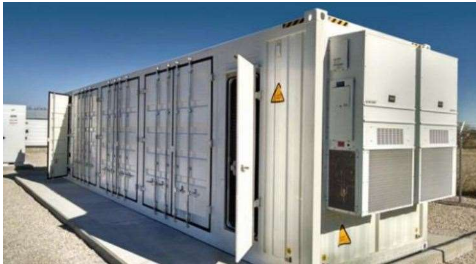
Figure 5-10 Representative Battery Storage System Enclosure (Exterior View)
