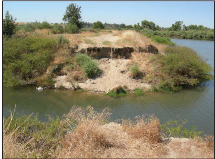
FIGURE 10: BREAK IN THE LEVEE DISCONNECTING SYCAMORE ISLAND FROM THE VAN BUREN UNIT.
